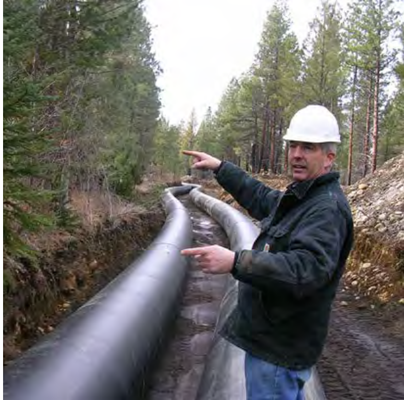
Deschutes Basin Partnership - Three Sisters Irrigation District Manager Marc Thalacker oversees canal piping, enabling flow restoration in the Creek.
