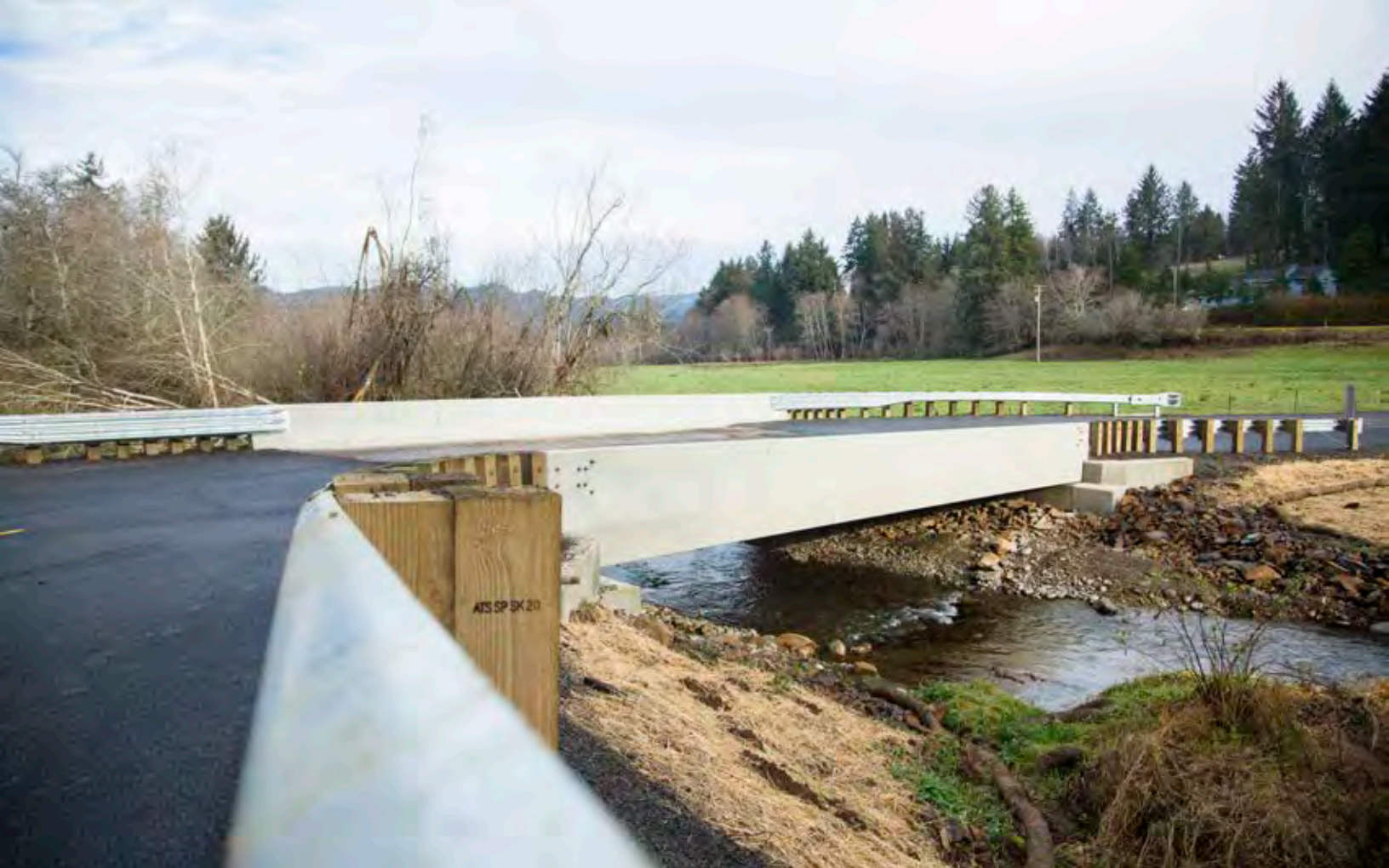
Salmon SuperHwy – A new bridge over Clear Creek, a tributary to the Nestucca River, and streambed reconstruction opened the watershed up for native fish use and natural stream function. Salmon were observed upstream of the bridge weeks after project completion. PHOTO / BRETT ROSS
