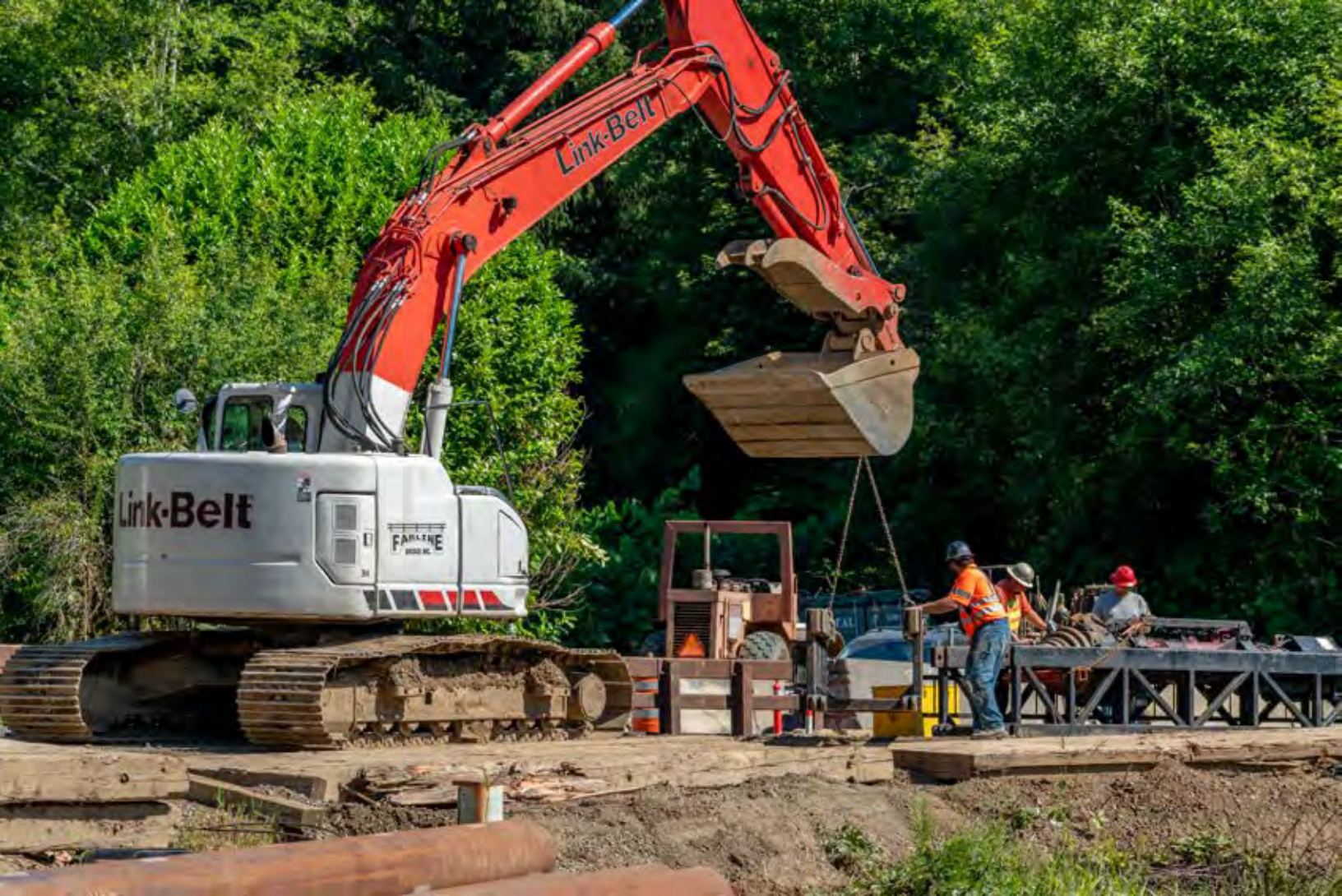
Salmon SuperHwy - Bridge construction on Peterson Creek to allow fish passage. PHOTO / TRAV WILLIAMS
